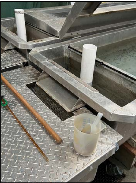
Outdoor (cistern) water is pumped into the first tank, then flows through a filter into the other tank.
